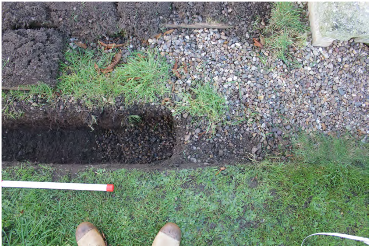
Plate 13 – northern end of Trench 01 looking south showing the point at which the trench met the existing French drain. Scale 0.5m, stone in upper right corner of frame is the north east corner of the chancel buttress.
