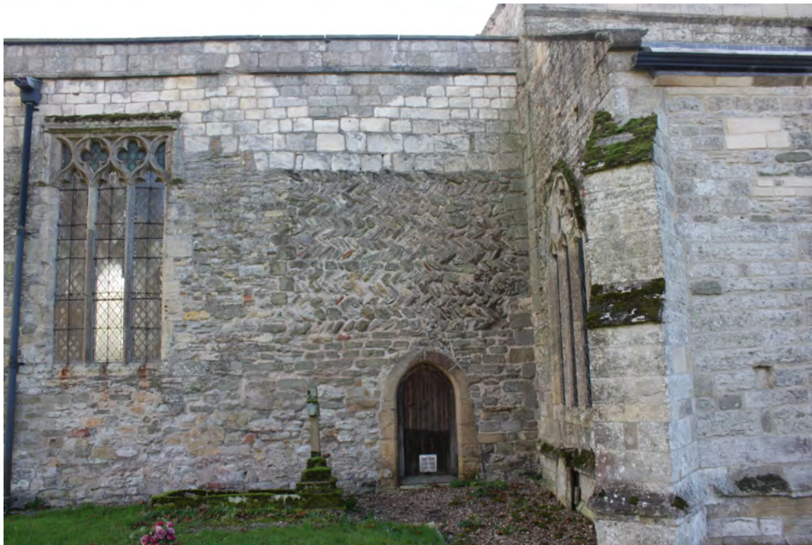
Plate 06 – herringbone masonry and orange tile in north chancel wall. Photographed looking south.
