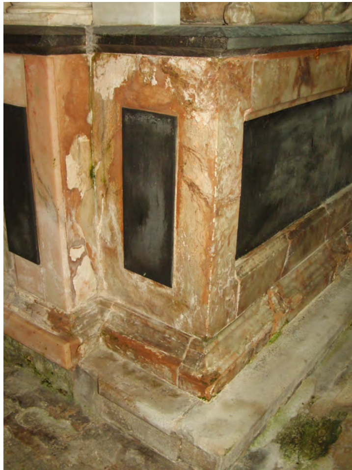
Plate 02 – water damage to the stonework of a monument in the church, also showing algal growth caused by damp conditions.
