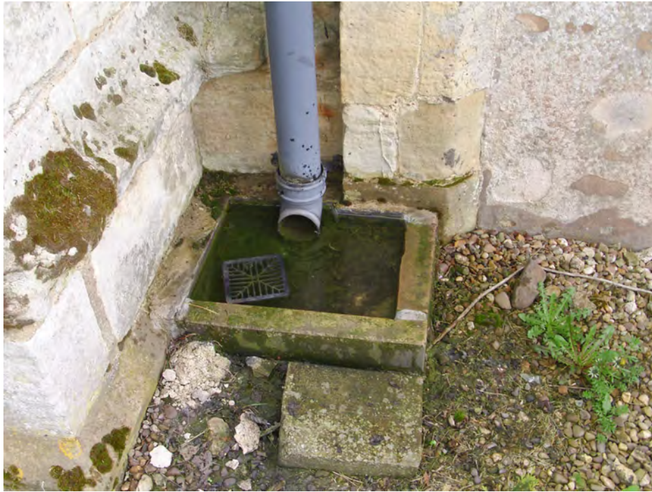
Plate 01 – standing water in drain beneath downpipe
