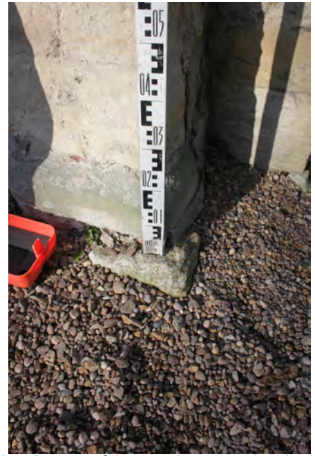
Plate 14b – close up of the TBM location, also showing gravel fill of French drain.
