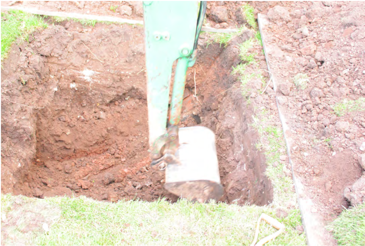
Plate 12 – excavation of soak away Pito1 showing depth of disturbed soil in base and very uneven sides. Looking east.
