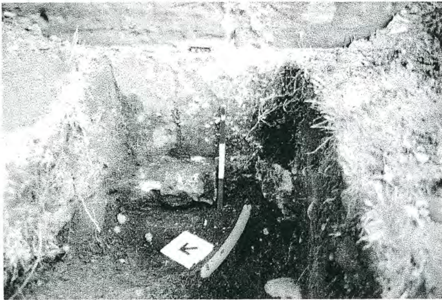
Plate 3: 05a, the partially exposed foundation of the tower with pipe inserted through the wall.
