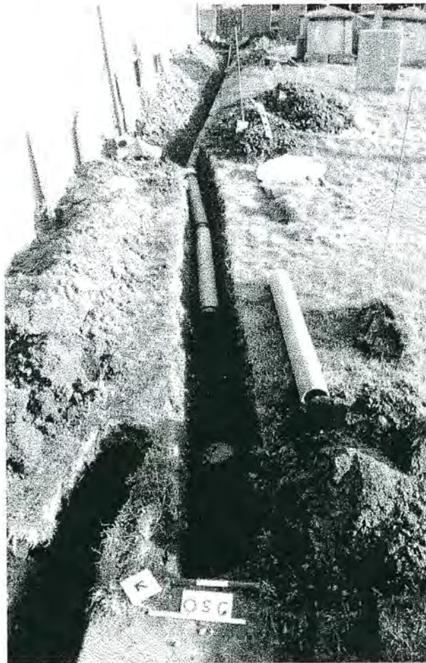
Plate 2: 02, the pipe trench running along the south side of the nave and chancel.
