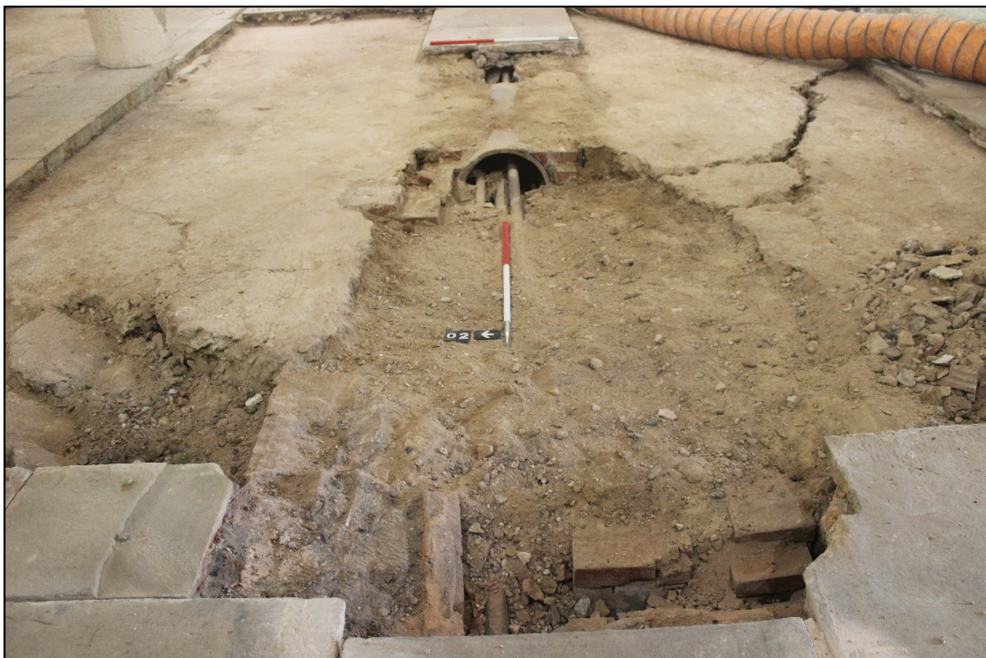
Plate 5: Heating pipe and trench in Area 02, the nave, viewed looking east. The brickwork in the foreground is later than that in the mid and background, a likely repair required due to subsidence which can clearly be seen in the lower half of the photograph.
